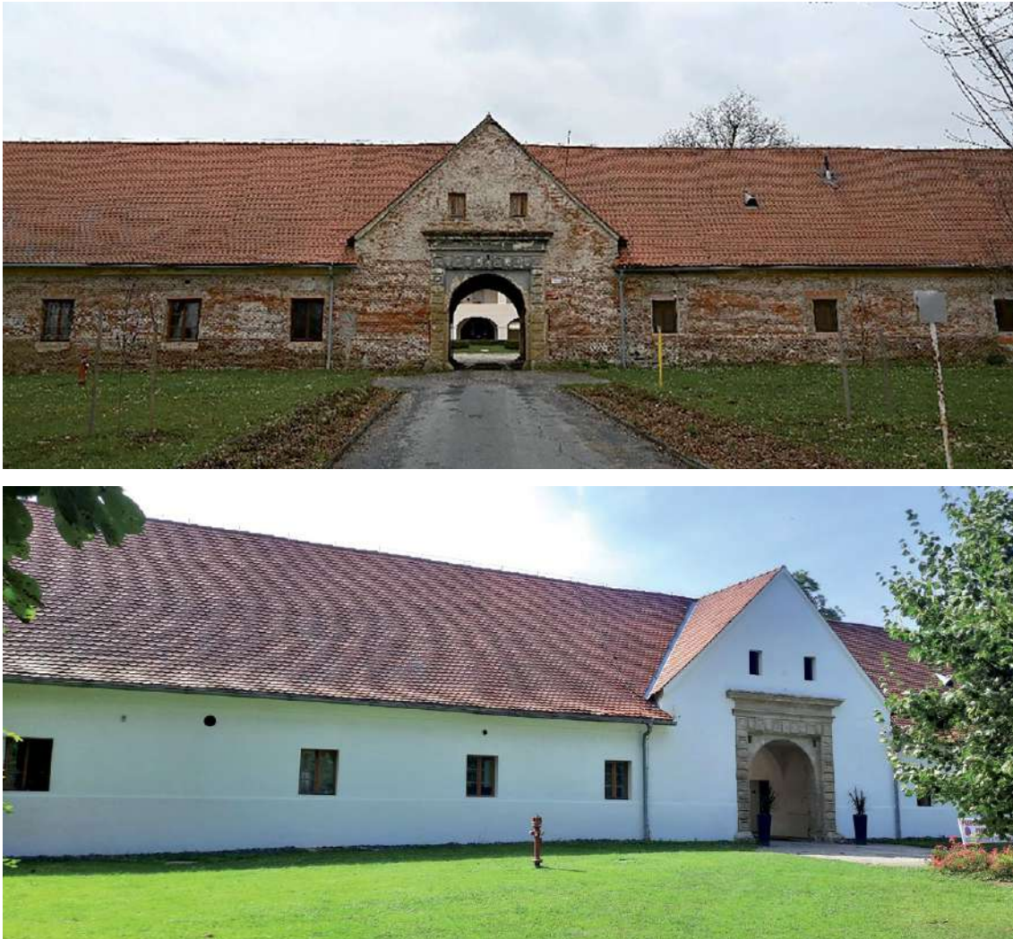
Fig. 8 Comparative photograph taken before the façade was restored, showing the bare structure of the building - the brick construction of the manor house, and later, when the façade has been completed and protects the construction of the building (photography by Tajda Benko).
