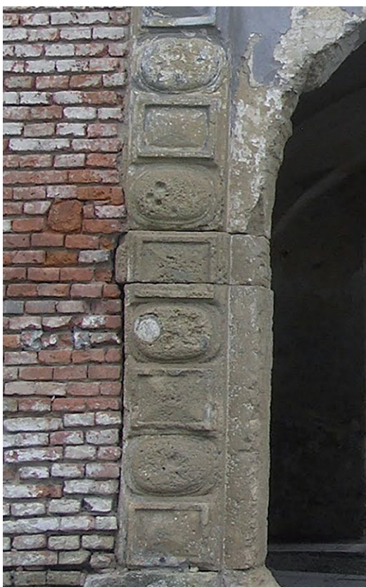
Fig. 6 Photograph of a single decorative field of the main portal of the Rakičan mansion prior to restoration, showing the stone structure and the base of the portal with an older grey coloured coating (photography by Tajda Benko).
